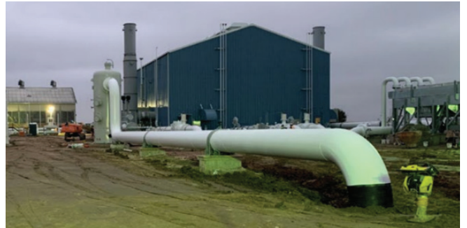
Ventura, Iowa, Compressor Building and Gas Scrubber.
