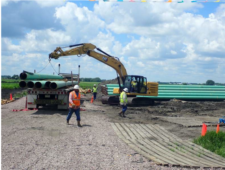
Facing northwest at MP 6.0, K & K offloading final load of FBE piping
