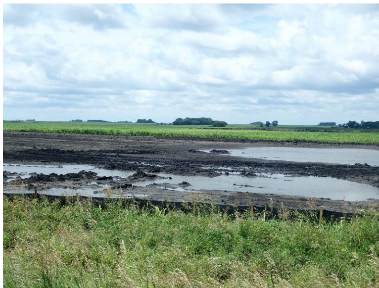
Facing west at MP 6.0, pipe staging area flooded due to excessive rainfall
