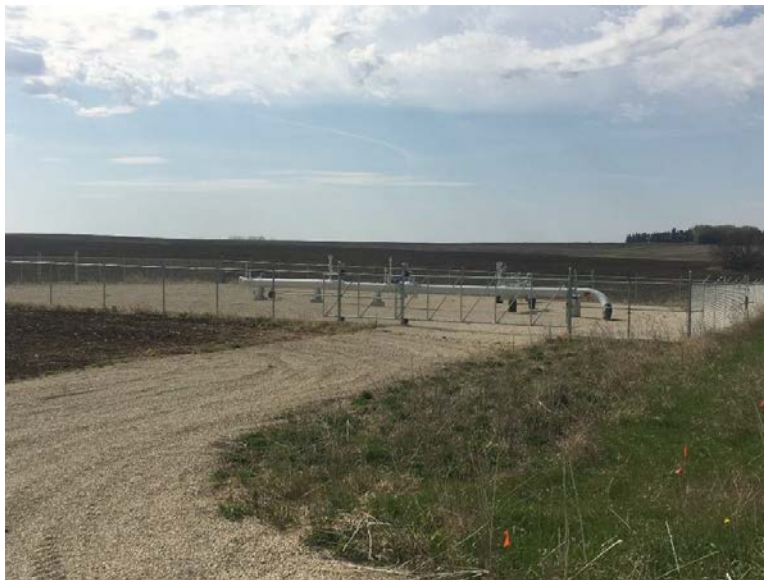
Facing south at MP 0.00, launcher station east of 95th Avenue SW, area stable and fully vegetated
