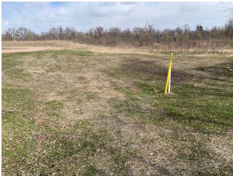
Facing northwest at the entrance to the Crow River HDD, 25% vegetative cover
