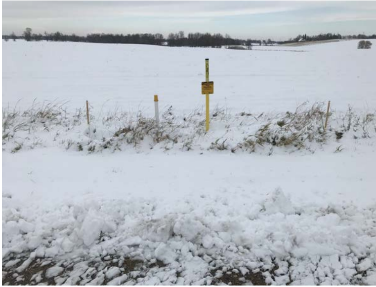
Facing north at MP 7.44, erosion control blankets (ECB) in roadside ditch north of Division Street
