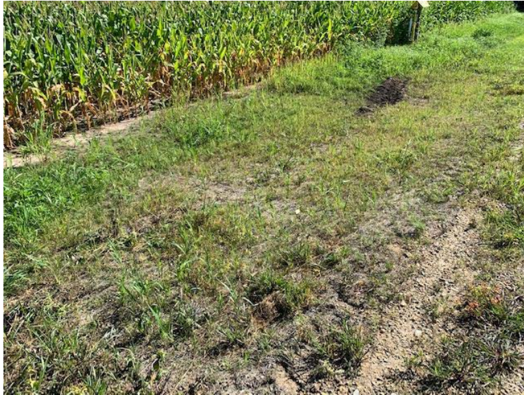
Facing northeast at MP 6.45, ECBs and vegetation impacted by landowner's tractor tires
