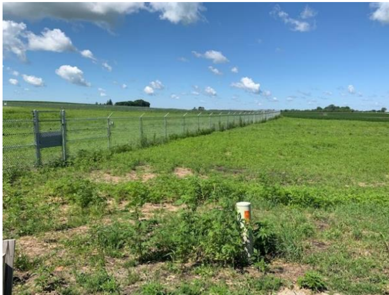
Facing southwest, seeded and mulched extra temporary workspace north of security fence, vegetation is progressing
