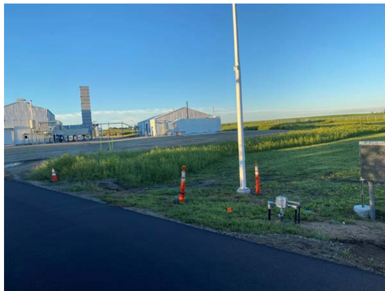
Facing west, infiltration trench is functioning properly and vegetation is progressing on banks of infiltration trench, driveway has been repaved
