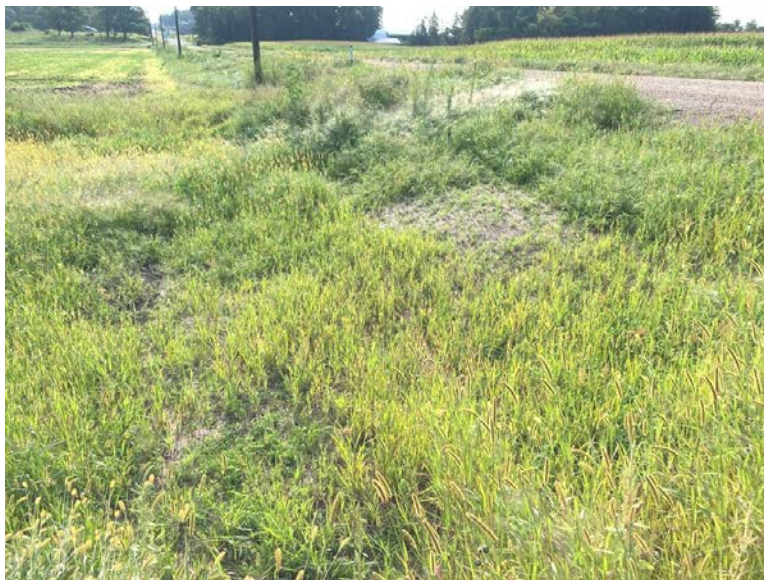
Facing east near MP 0.1, north side of 134th Street, ECBs in roadside ditch, vegetation has reached 65%
