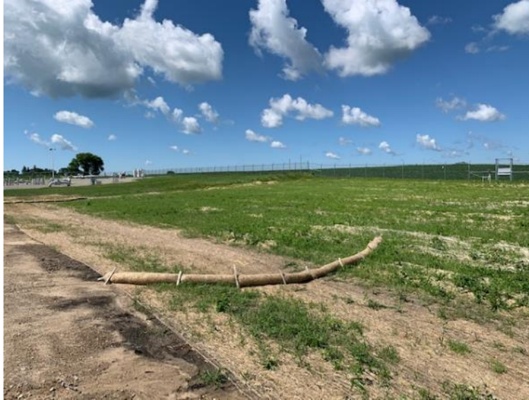
Facing southwest, ECB installed along slope and over drain tile trench west of compressor station auxiliary building, vegetation is progressing
