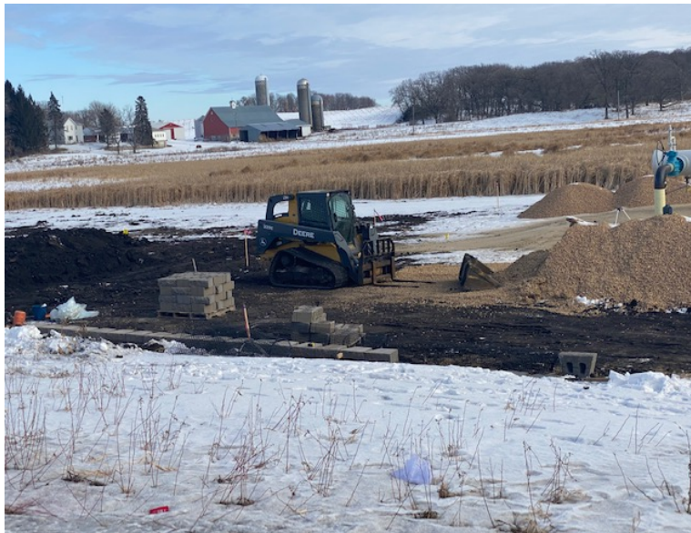
Facing southeast at MP 0.0, Minnesota Limited preparing to grade soil for interior of retention wall
