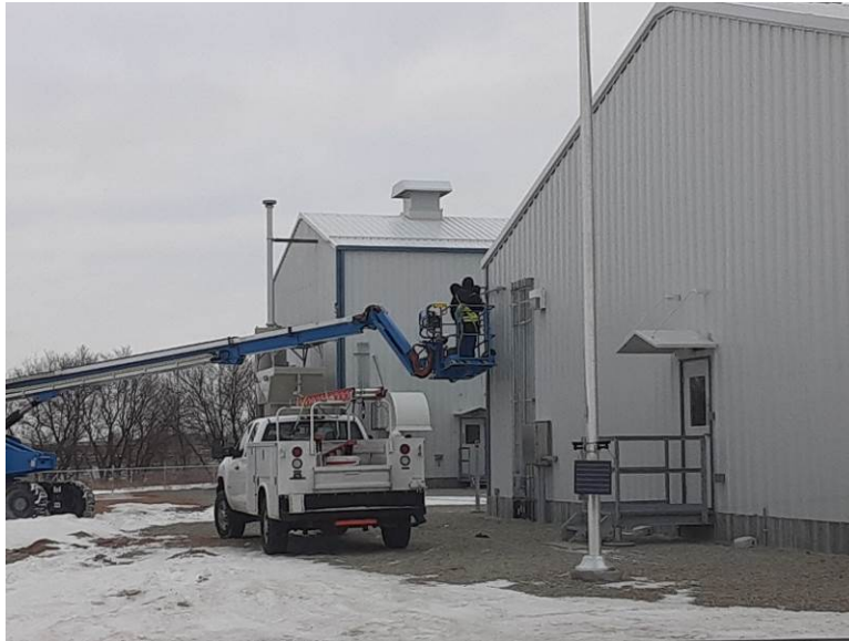
Facing east, ASI installing security camera on north side of the auxiliary building
