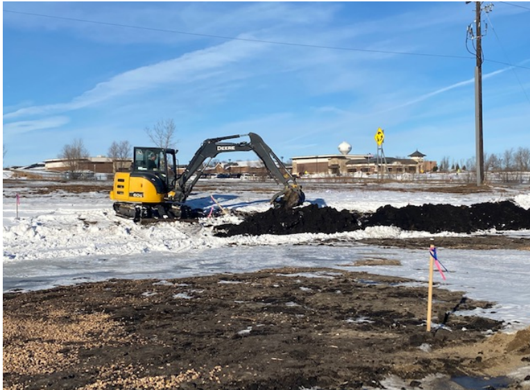
Facing north at MP 0.0, Minnesota Limited excavating trench for retention wall east of 134th Street
