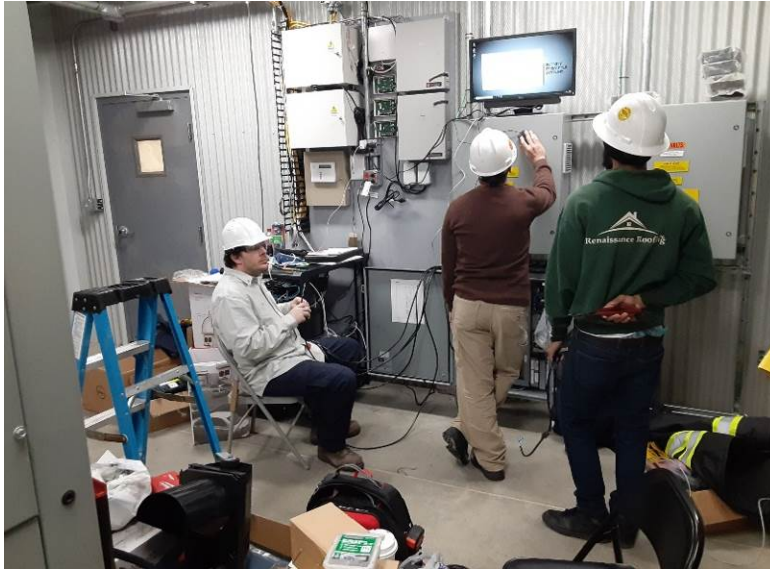
Facing southwest, ASI terminating wiring and programming security system in the control room
