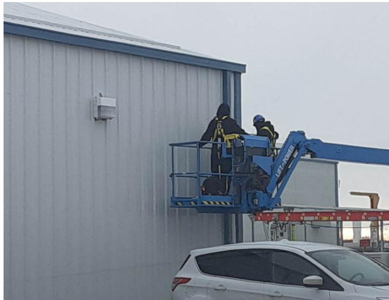
Facing southeast, ASI installing security camera on south side of the auxiliary building
