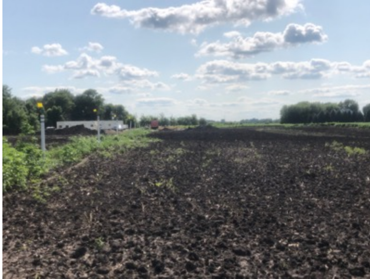
Facing southwest at MP 0.1 north of 290th Street, topsoil has been restored
