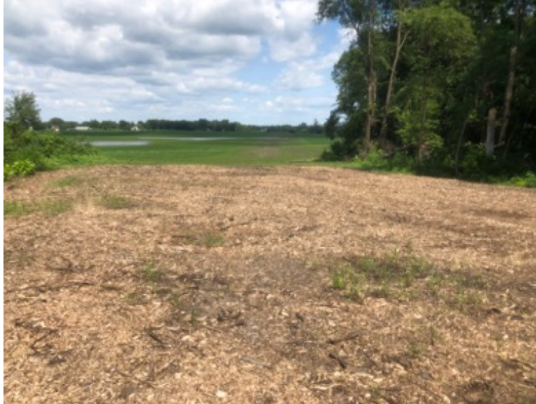
Facing northeast at MP 0.8, area cleared of trees, seeded and wood mulched; field in background planted with soy beans by landowner
