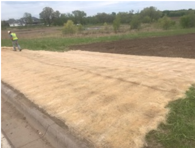
Facing west, MP 0.1, access to the construction yard along 132nd Street W, seeded with MN DOT ditch mix and stabilized with erosion control blanket
