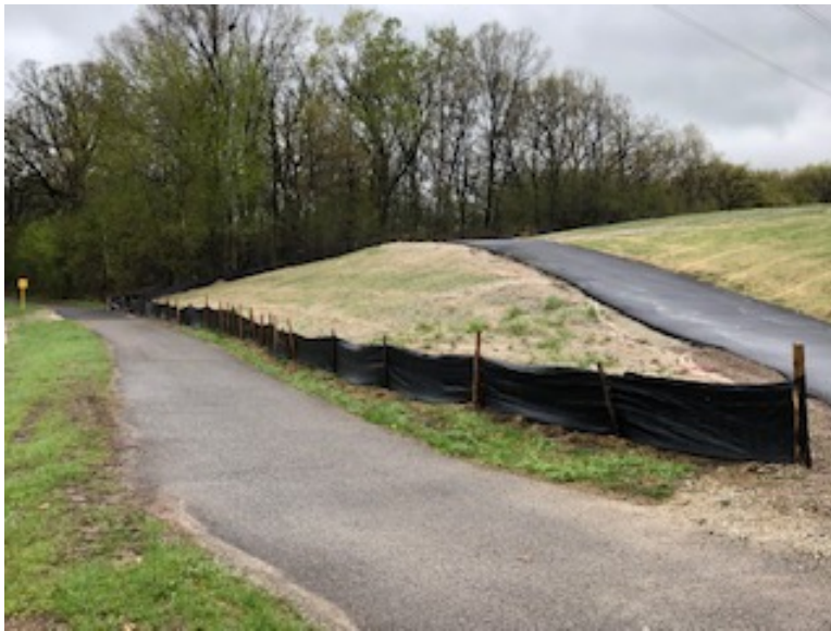
Facing south, MP 4.8, along Thomas Lake Road, Minnesota Limited intends to sub-contract to a paving company to replace the bituminous trail
