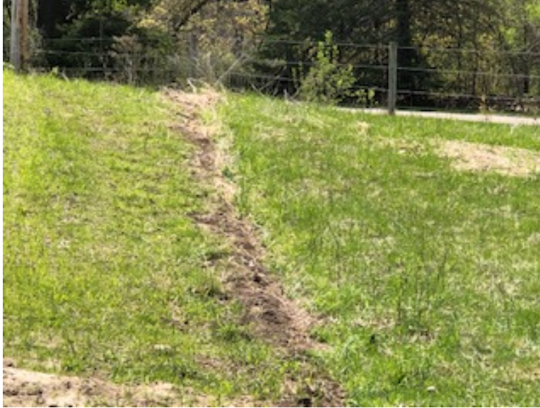
Facing east, MP 1.9 near Chinchilla Avenue, vegetation reached 70% and silt fence was removed
