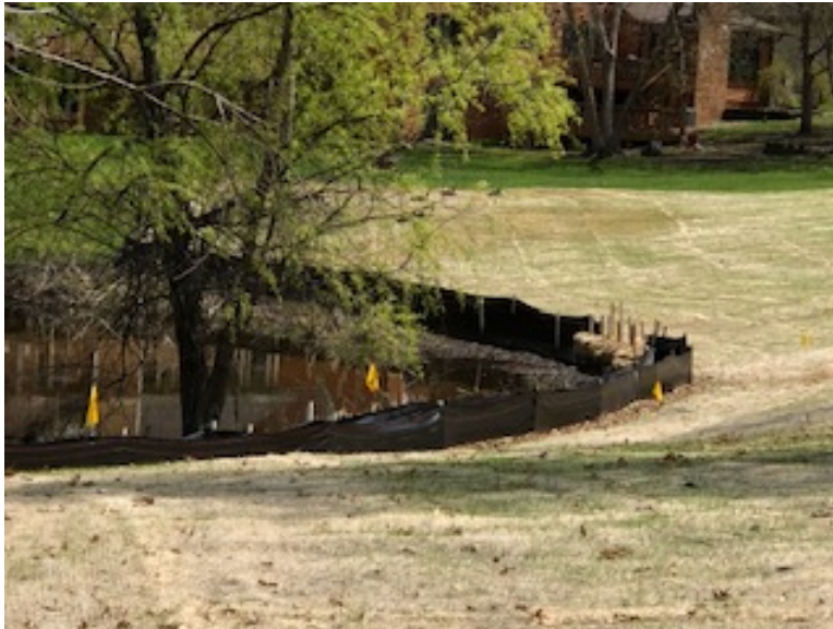
Facing east, MP 4.3, redundant silt fence protecting wetland DA-079; area is at approximately 50% revegetation
