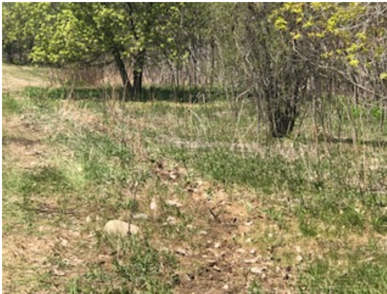
Facing north, MP 7.0, off Cedar Ridge Circle, north side of extra temporary workspace, vegetation reached 70% and silt fence was removed
