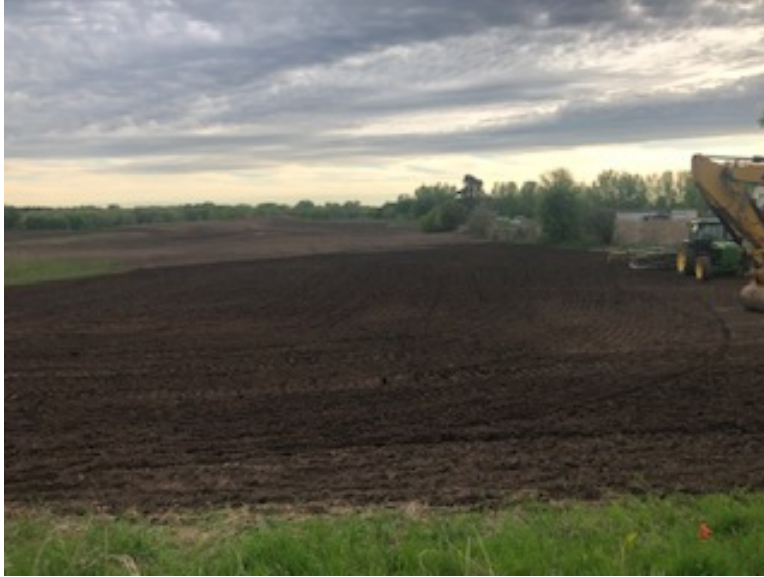
Facing north, MP 0.1 to MP 0.3, the contractor restored the staging area and returned the land to agricultural use
