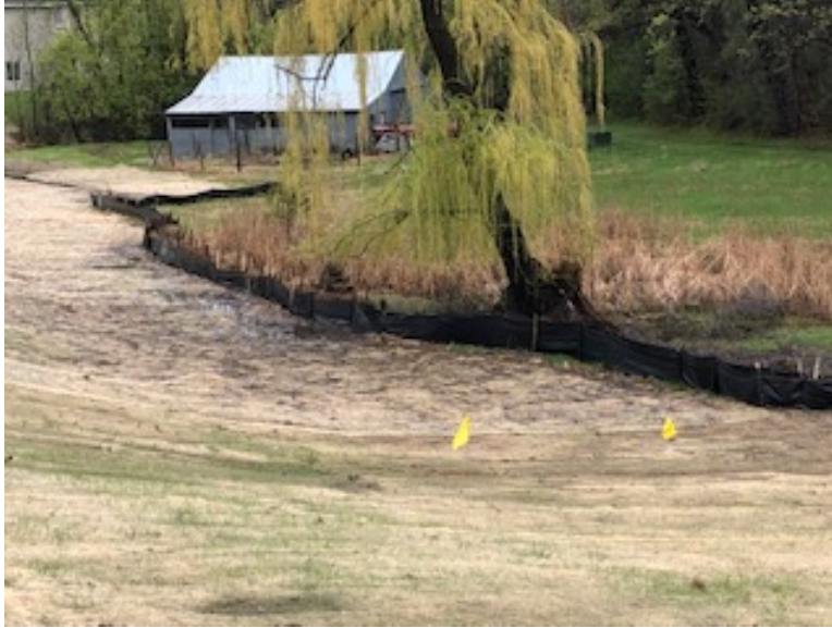
Facing north, MP 4.4, redundant silt fence protecting wetland DA-080 along Thomas Lake Road; the area is at approximately 40% regrowth
