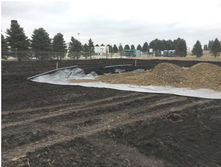
Facing southeast, Heselton commenced installing geo-tech fabric and rock for access road
