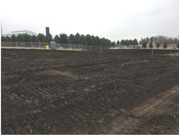
Facing southeast, Heselton Construction, LLC, (a subcontractor) commenced topsoil removal for staging area
