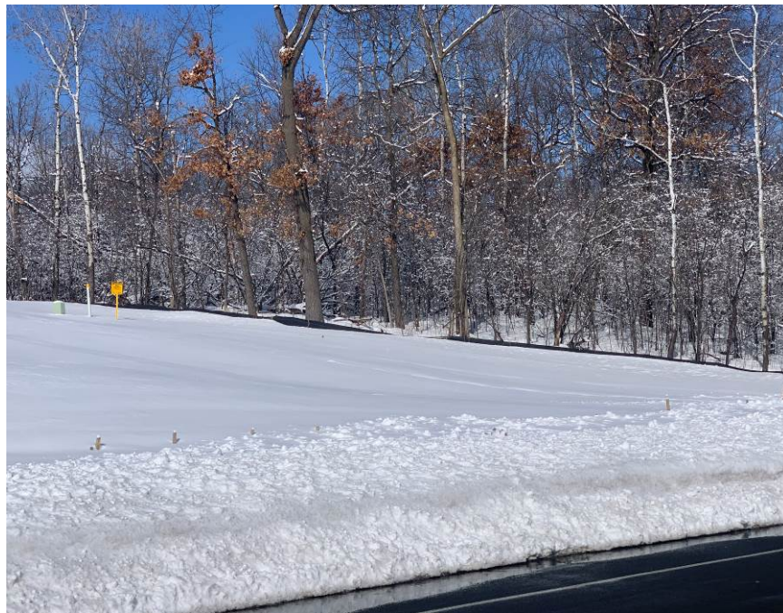
Facing northwest at MP 4.8, west of Thomas Lake Road, perimeter silt fences covered by snow along the road and along the wood line
