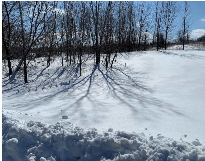
Facing southeast at MP 4.4, silt fence covered by snow east of the private drive
