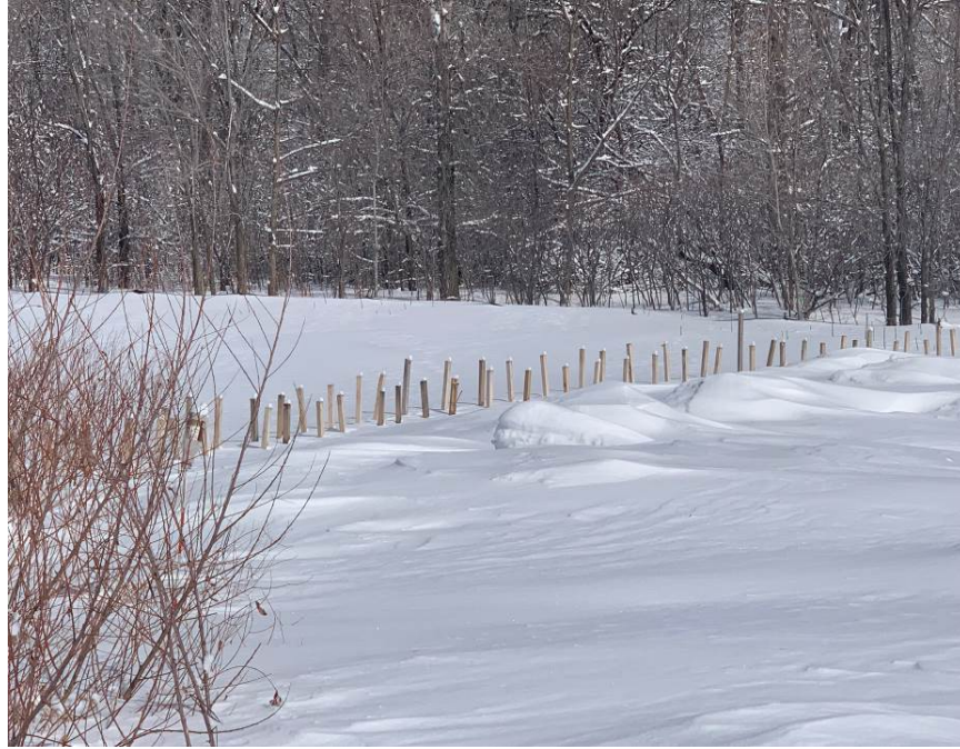
Facing northeast at MP 7.0, straw bales covered with snow north of Cedar Ridge Circle
