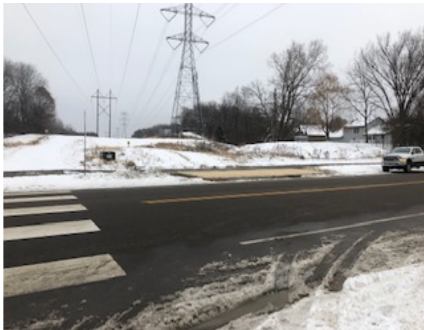
Facing west, MP 6.5, Sandstone Rd., seeding and curb completed, inspection found no erosion
