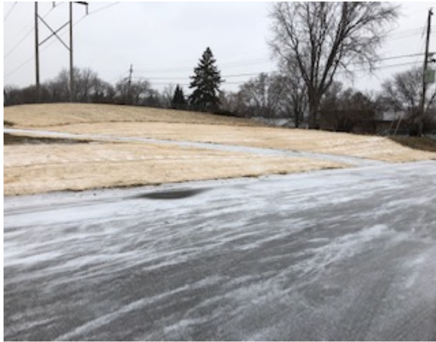
Facing west, MP 5.3, Johnny Cake Ridge Rd., seeding completed, inspection found no erosion
