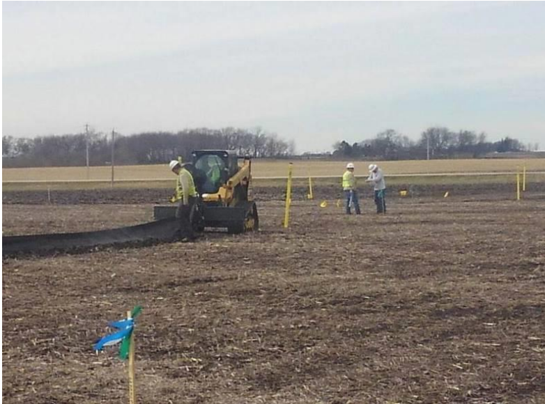
Facing northwest, contractor commenced installation of silt fence for Wetland OCS-W1 buffer
