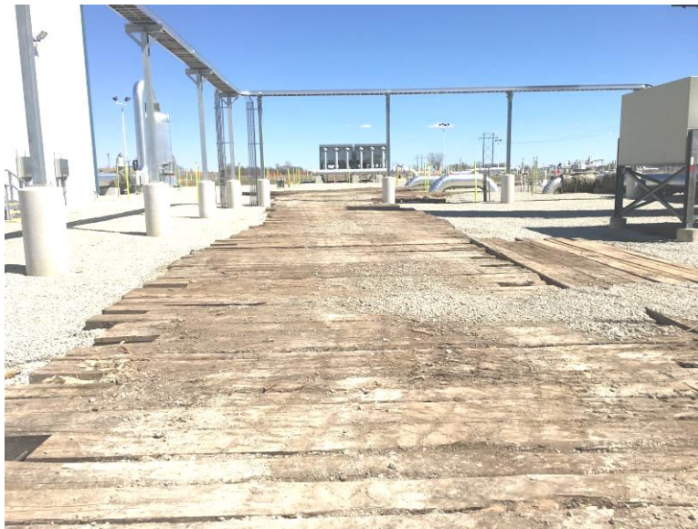
Facing east, commenced installation of timber mats for the travel lanes inside the existing compressor station yard
